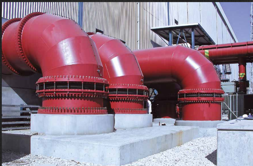
Lateral expansion joint type U110M in the cooling water system of a coal-fired power plant. NB 2600, 4 bar
