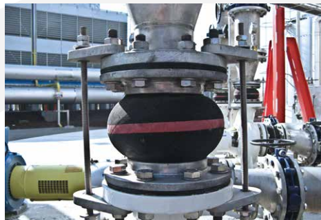
Lateral expansion joint type U110R on the pump pressure side of a lye pipe in a paper factory. NB 125, 5 bar ▶ page 17
