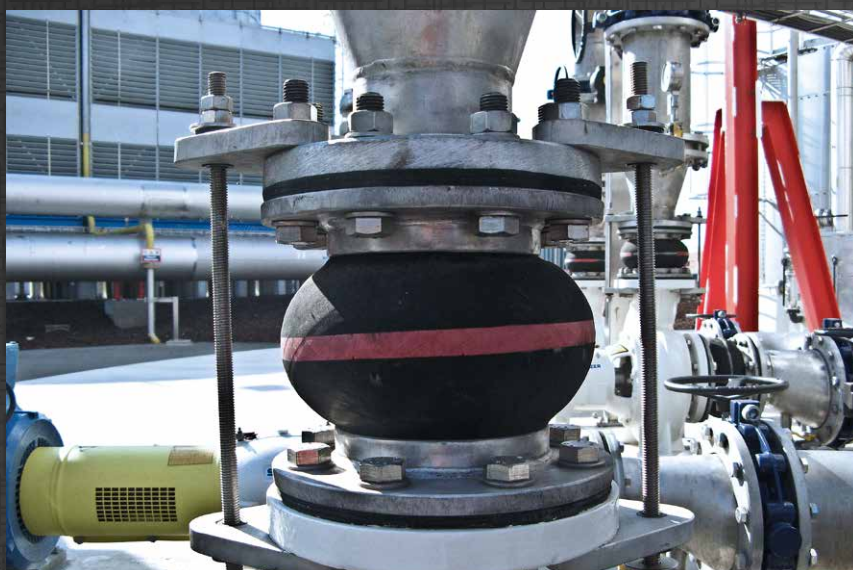
Lateral expansion joint type U110R on the pump pressure side of a lye pipe in a paper factory. NB 125, 5 bar
